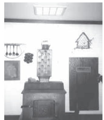
A large vent in the ceiling directly above stove leads to a 20-in. sq. fan box in attic.
