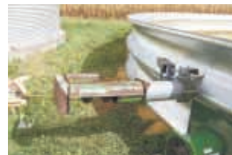
He cut a hole in the side of rings used as retaining walls, running the auger to the center of bin.
