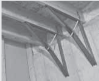
CornerCam is used at truss ends to strengthen and straighten sagging joists.
