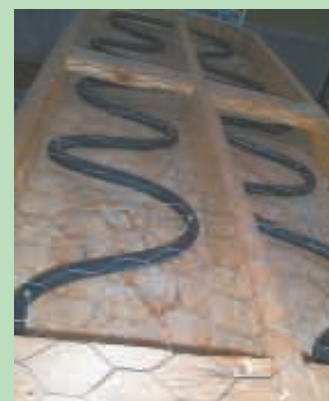
Compost-heated water runs through lengths of insulated hose under growing tables in greenhouse.
