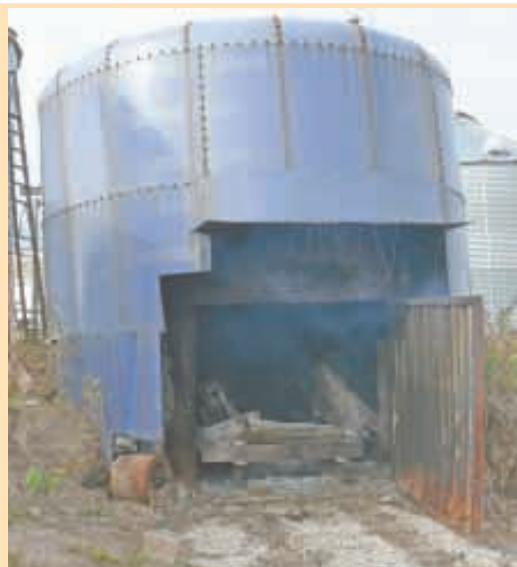
Stortz put a section of a 28-ft. Harvester silo over the 24-ft. dia. firebox.
