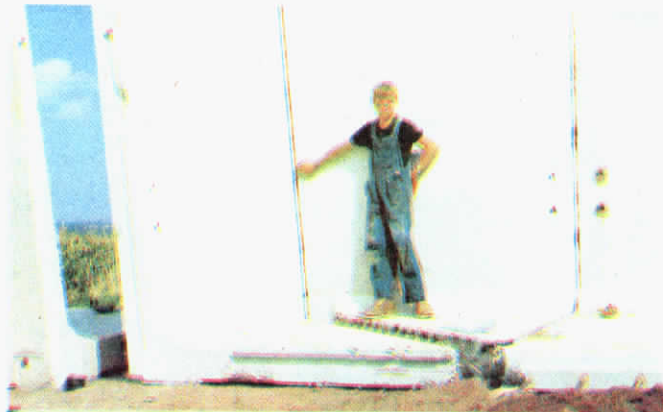
A solid flat base is built up with about a 2 in. grade to allow silage acids to drain out of the silo. Wall sections are 4 in. thick at top, 8 in. at bottom.
