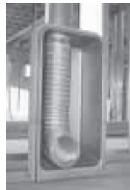
Receptacle holds vent hose in wall behind dryer.
