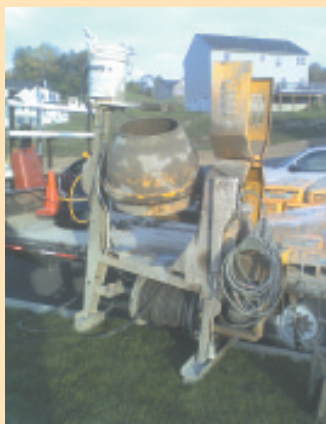
Hose reel under concrete mixer hooks up to faucet on house. It fills a 5-gal. bucket on top of mixer, which releases water into mixer's drum.
