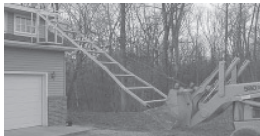
Cherry picker attaches to bucket on Eilers's Case backhoe and will lift up to 25 ft. high.
