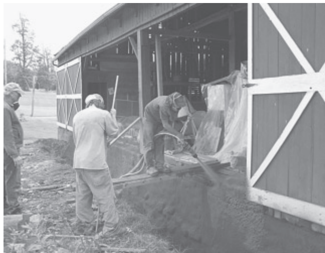
Pneumatic pressure is used to force dry concrete, sand, and Portland cement through a hose, with water injected just before application.
