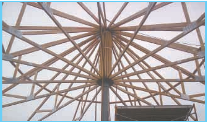
An 8-in. dia. vertical steel pipe runs up middle of structure and is used to support custom made trusses, which rest on a thick steel plate welded to pipe.
