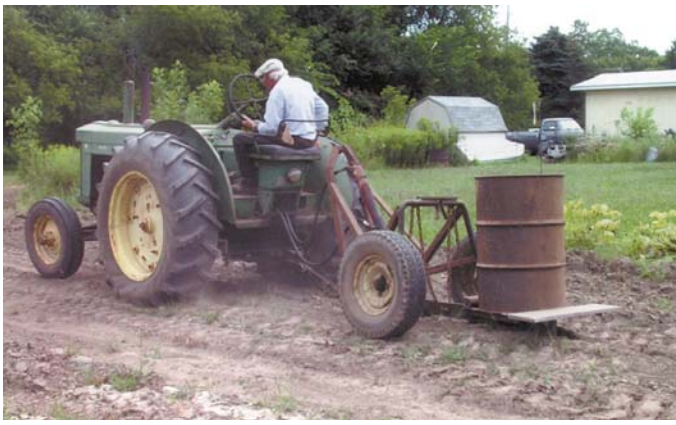
Bernard Belanger uses a pull-type subsoiler to put a 4-in. dia. row of pea rock about 24 in. under the ground. "It's quite a bit cheaper than using tile," he says.
