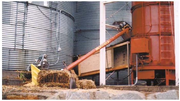
Dryer fan on other side of holding bin pulls air through wooden ductwork into dryer.
