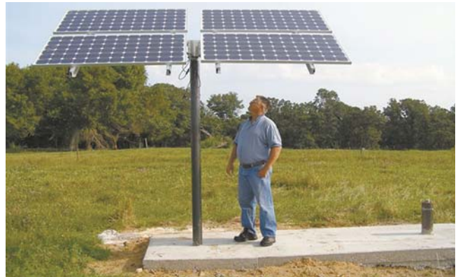
Paul Heers uses a solar panel and pump to deliver water through an underground pipeline to six 900-gal. tanks.
