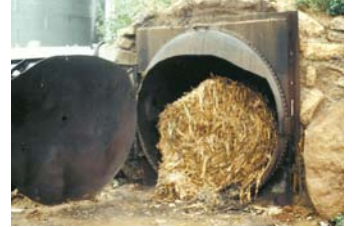
Furnace is built out of an old asphalt boiler, with a door cut into one end.
