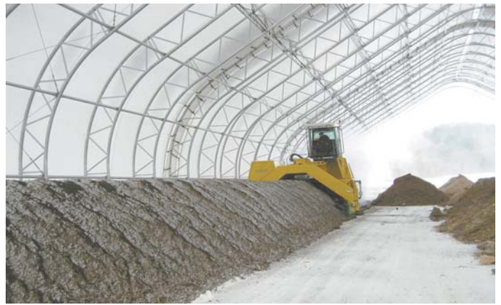
One week's worth of manure is enough for one windrow in the 100 by 250-ft. composting buildings.
