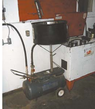
Funnel mounts on top of pipe to catch used oil under car lift, with the oil draining into an air compressor tank.
