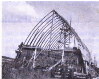
Poles run all the way from ground up to a ridge pole on top. Bonnett built hay loft inside and nailed roofing boards to poles.
