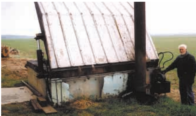
To heat their huge 120-ft. sq. shop, Clair Wilson and his sons built a giant wood-burning furnace into an embankment next to the shop.
