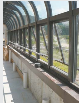
Cool air is brought back to front side of greenhouse through pvc pipes. After the air is reheated it’s recirculated back underground.
