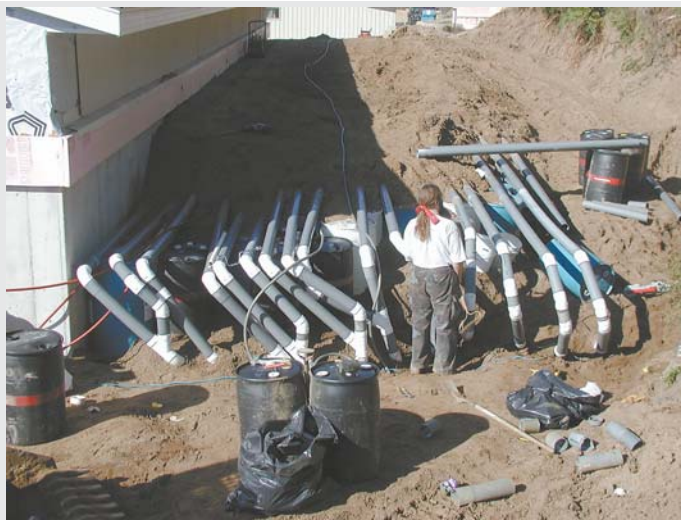
Heat is transported from the greenhouse to the buried barrels by 2,600 ft. of 4-in. dia. pvc.
