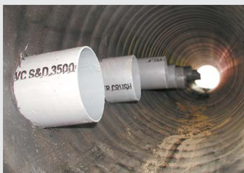
A manifold made out of 15-in. dia. plastic culvert distributes heat to the pvc heat pipe.
