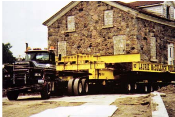
Sheets of 4 by 8-ft. plastic have many uses. Here a house-mover has laid sheets beneath a truck's wheels for use as a temporary roadway.
