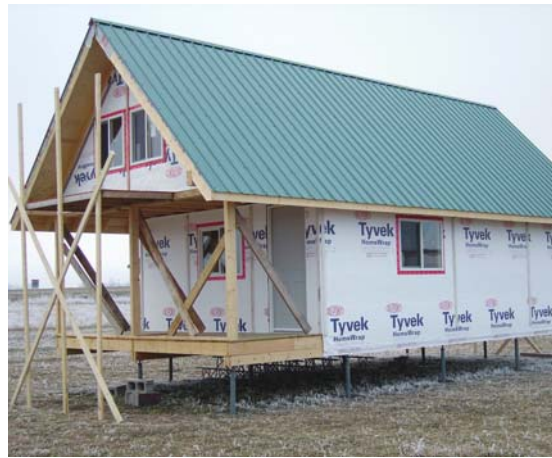
Cabin’s floating foundation uses telescopic posts and air-over-hydraulic jacks, permanently bolted to wooden beams, to raise building up before water arrives.
