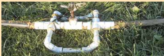
Homemade sprinkler pad consists of a pair of 1 1/2-in. pvc cross fittings, with a sprinkler mounted between them, and 1-in. runners to either side.
