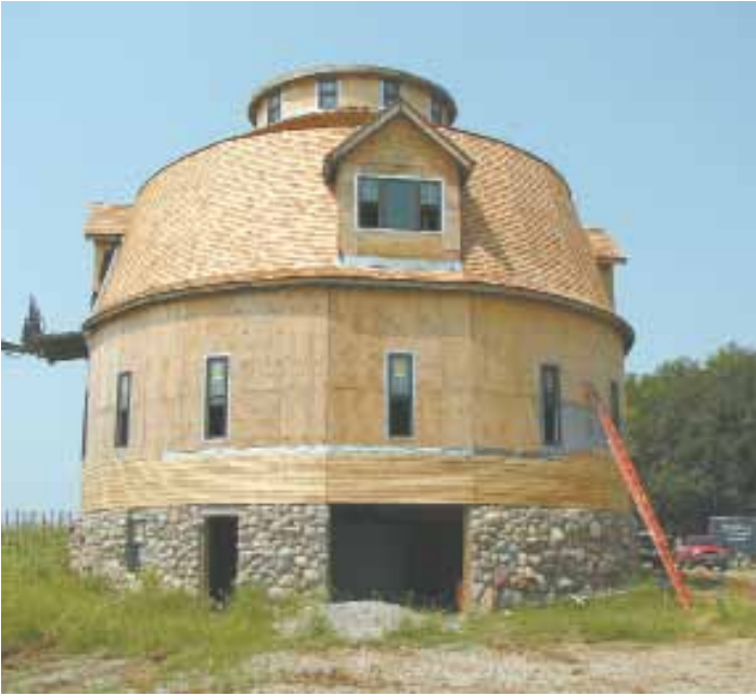
Bruce Willemsen remodels older barns and builds new barns based on older styles. His latest project - a big round barn - is proving to be an interesting challenge.
