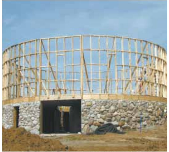
The built-from-the-ground-up round barn has a root cellar and garage at the bottom, and a wood shop and canning kitchen on the next floor.
