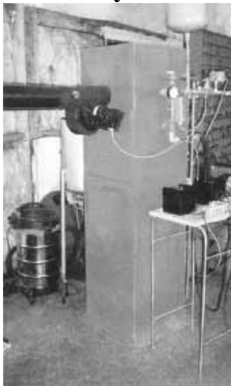
LST pellet stove and hot water boiler burns hay and wood pellets, as well as corn. It eliminates naturally forming clinkers that might smother fire.
