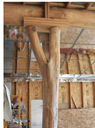
Struble selected Y-shaped logs for internal support posts, fitting the top with support plates.
