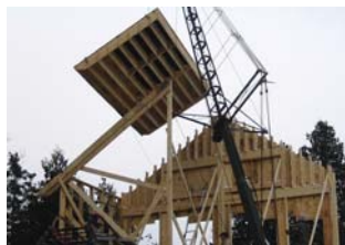
Even the roof was pre-fabbed in panels that could be lifted into place.
