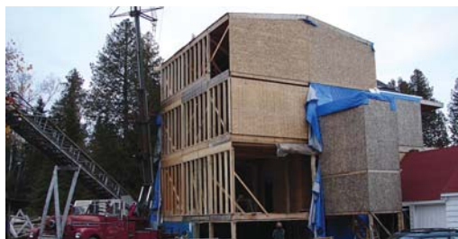
Jim Struble prefabricated this multi-story, 4,500 sq. ft. house himself, assembling it in 3-story segments on the ground. House is shown here nearly complete.
