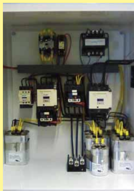
Photo shows Remco's 480V automatic rotary phase converter panel equipped with multiple irrigation pump controls for additional loads.
