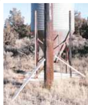
After setting this post in the ground, Knoche used his homemade T-post "spade props" to keep post absolutely vertical.
