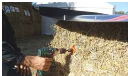
Wire rope "loops" at each end are used to secure cap to bale. You stretch loops down tight and then insert plastic screw-in anchors into bale with a cordless drill.
