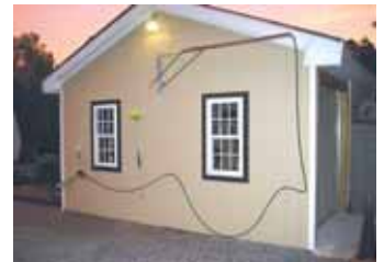
A 10-ft. long pivoting hose arm mounts above one of the garage windows.
