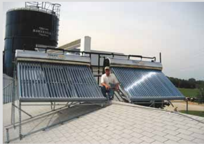
Tom Trantham installed his American Microsolar rooftop hot water heater last winter and says it already has saved him $200 a month in reduced gas bills.
