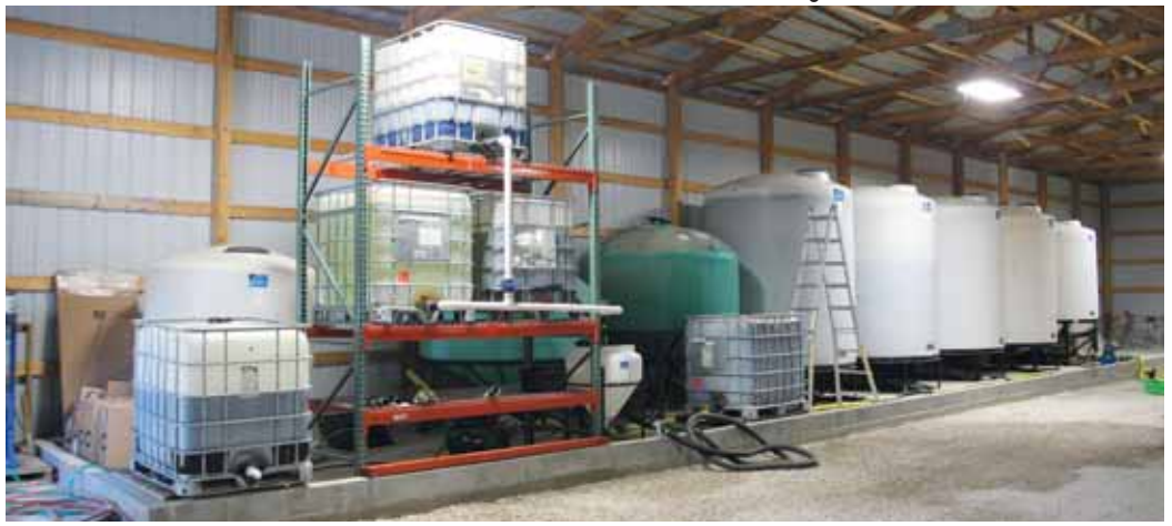
The 104-ft. long containment chamber, made of reinforced concrete, contains all the Rengers' liquid fertilizer products and farm chemicals. A rack holds totes.
