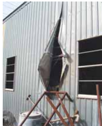
James Kelley woke up one morning to find a hole ripped through the sheet metal siding on his farm shop. It was caused by an air compressor explosion.
