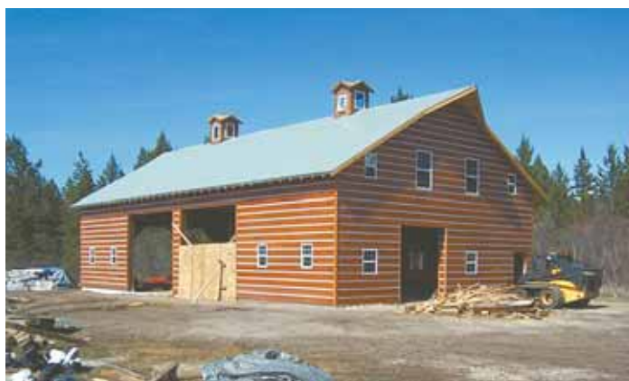
Relocated barn got a new metal roof, custom siding with a chinked look, and 2 new cupolas.
