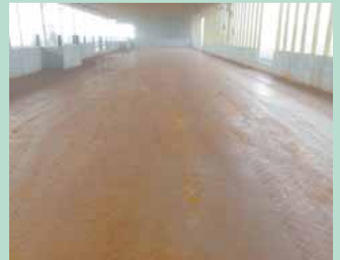
Cattle barn floor treated with Perma-Zyme. After raising 250 steers to market weight and cleaning it out, the floor was still solid.
