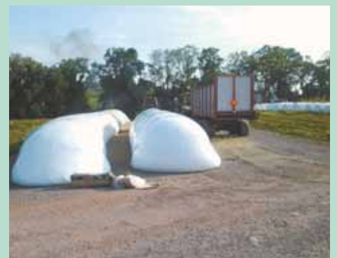
A dairy operation used Perma-Zyme to make a 50 by 220-ft. pad for silage bags. The site was chiseled and Perma-Zyme mixed in with a disc. A culti-mulcher was used to level the site and a vibratory roller provided needed compaction. Dairyman Bobby Waite says the surface has held up solidly to many daily trips by tractors and skid steers.
