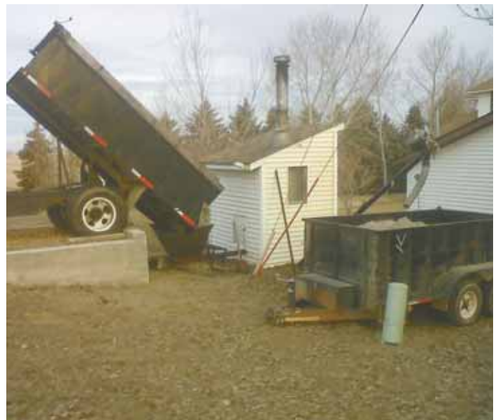
Gooseneck trailer dumps into outside hopper with auger that feeds furnace inside. Ashes are augered out into a second trailer for disposal.
