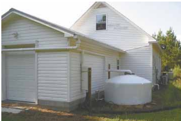
Another 1,100-gal. tank outside collects water from rain gutters fitted with microscreen filters and a first-flush diverter to take out debris before going into the tank.
