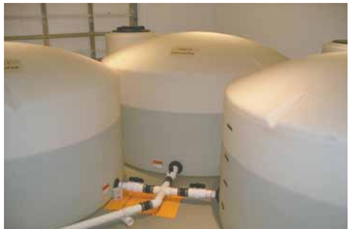
When Mike Minga built his home, he included a 24 by 25-ft. room to hold four 1,100-gal. tanks and the necessary pumps and filters to provide water to the home.
