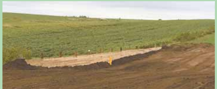
Fences are designed to hold water until it drains into standpipes. Fence shown above is 130 ft. long, with 8-in. posts spaced 10 ft. on center.
