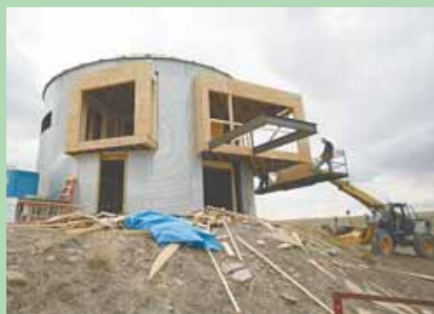
One set of living room windows look inside at the curved wall of the bin, and the others are on the bump out to capture the outdoor views.
