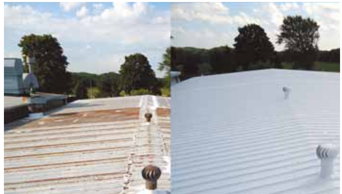
Luke Schweitzer uses rubberized coatings in his roof-coating business, providing a waterproof membrane that repairs leaks and greatly extends roof life. These are before and after photos.
