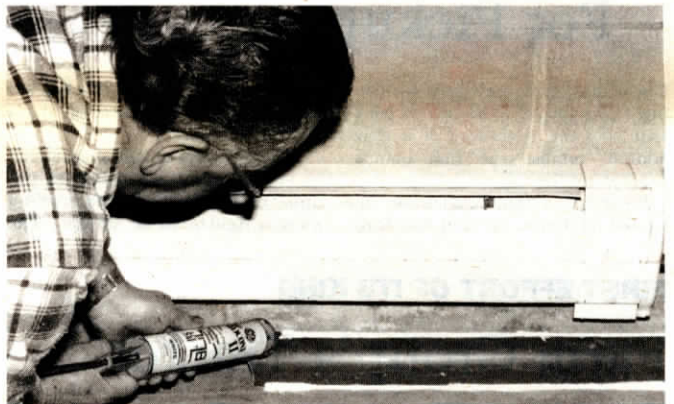
Silicon caulking along the top and bottom of the pipe strips forms a water-tight seal.
