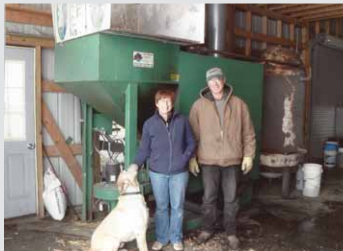
The Franzenburgs use a high output Year-A-Round corn burning furnace to heat greenhouses equipped with radiant floor heating.
