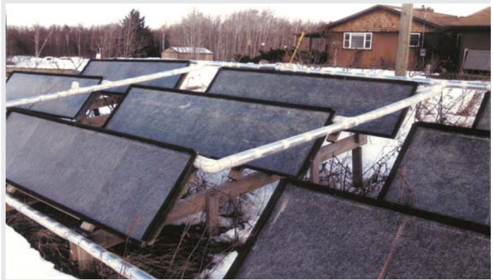
Fifteen 2 by 8-ft. solar collectors provide hot water heat for Joseph Rupinski's home.
