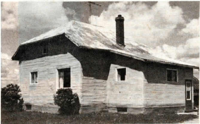
Canadian farmer Victor Genier, of Cochrane, Ont., sprayed his farm home - roof and all - with a thick layer of insulation to protect against winter winds and sub-zero temperatures.
