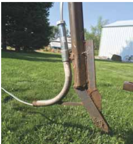
A curved 1-in. dia. tube clamps on behind 3-pt. trencher to feed cable down into trench.
