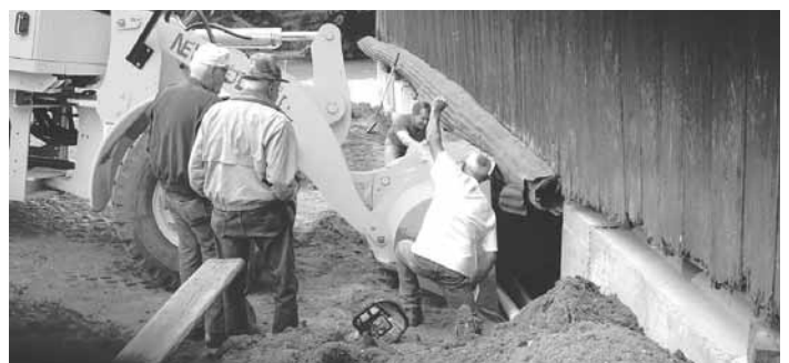
The entire project took 5 years, starting with a concrete foundation at one end of the barn where members used a big loader to push 3,800-lb. concrete blocks into place.
