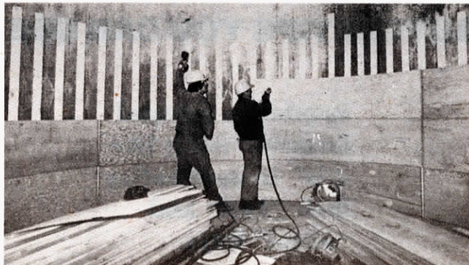
Crews essentially build a barrel inside the silo by nailing 1 by 4's directly onto silo walls, then stapling on 1/2 in. plywood or Blandex liner. Base price for converting a 20 ft. dia. silo is 45 to 50 cents per bu.
