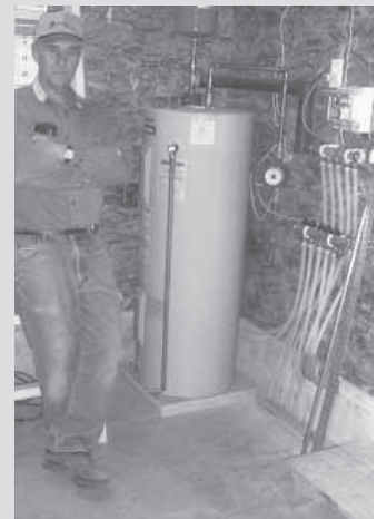
The system has two sets of manifolds, one for pipes going out and one for returning, and manifolds where you control the flow from the water heater.
