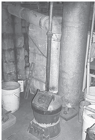
Water circulates from 30-gal. reservoir to “bucket-a-day” wood stove and then back into reservoir. Water is pulled from the reservoir by hot water heater as needed.
