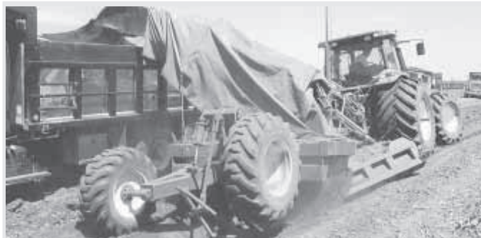
Miller used this 8-ft. Liebrecht rotary ditcher to clean out road ditches that had filled up with soil from nearby fields. The work was part of a highway improvement project.
