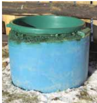
Filler material is inserted loosely into space between tubs to within 6 in. of the top. Then spray foam is applied one layer at a time, allowed to cure, and spray painted.
