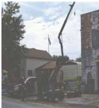
Remote control, 2,000-lb. electric winch mounted at top of crane does the lifting.
