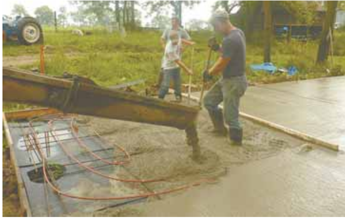
When Matt Eby built a new workshop, he saved time and money by drilling holes for concrete piers and filling them with concrete at the same time as he poured the floor.
