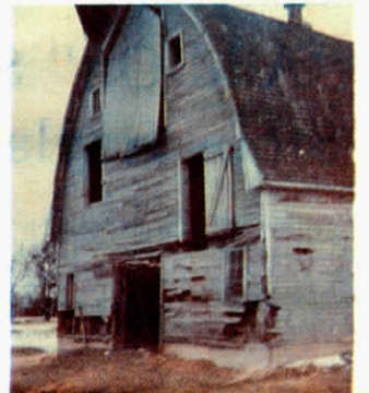
Bottom 6 ft. of the old barn was cut off and the remaining portion lowered to the ground.
